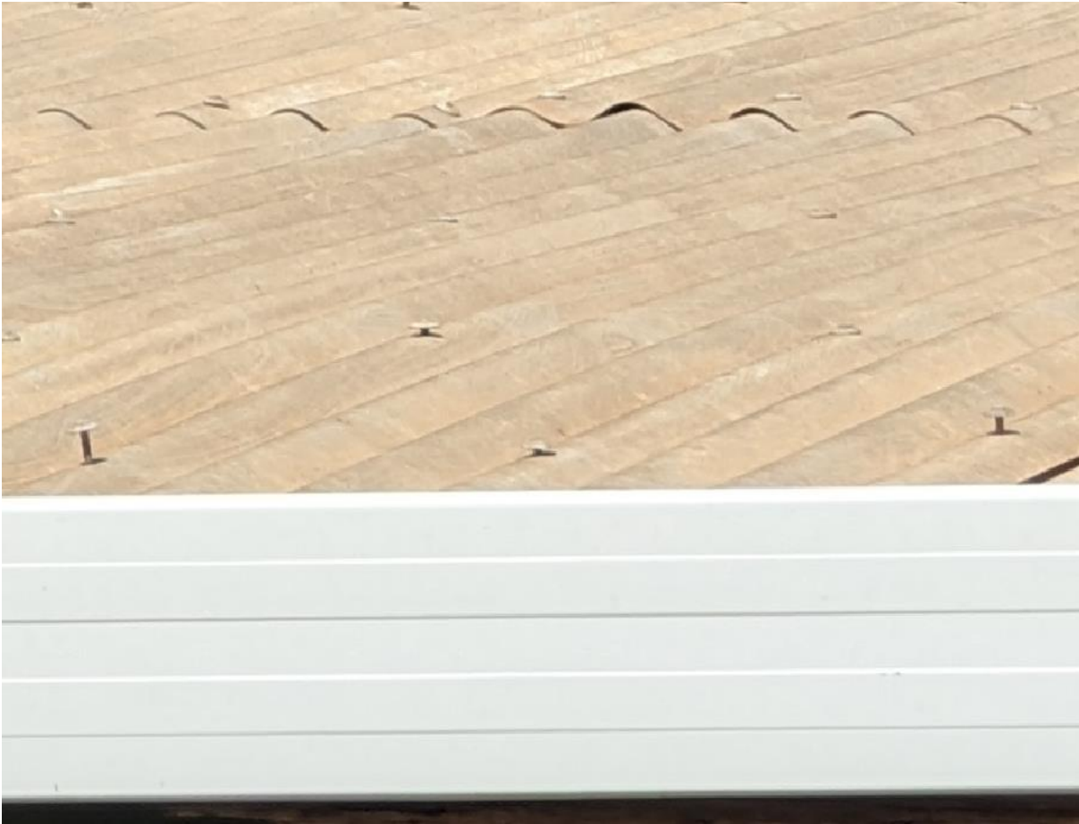
Figure 17: Roof sheeting nails lifting.
