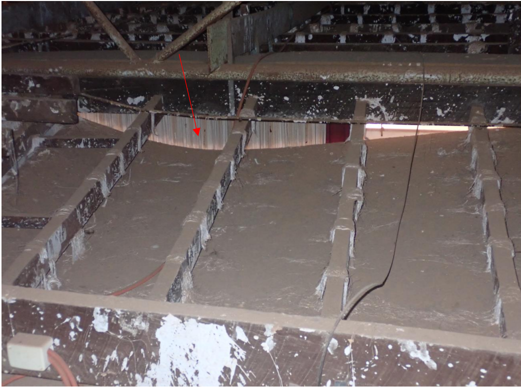
Figure 9: The horsehair plaster fixing ceiling and joists has let go in some areas.
