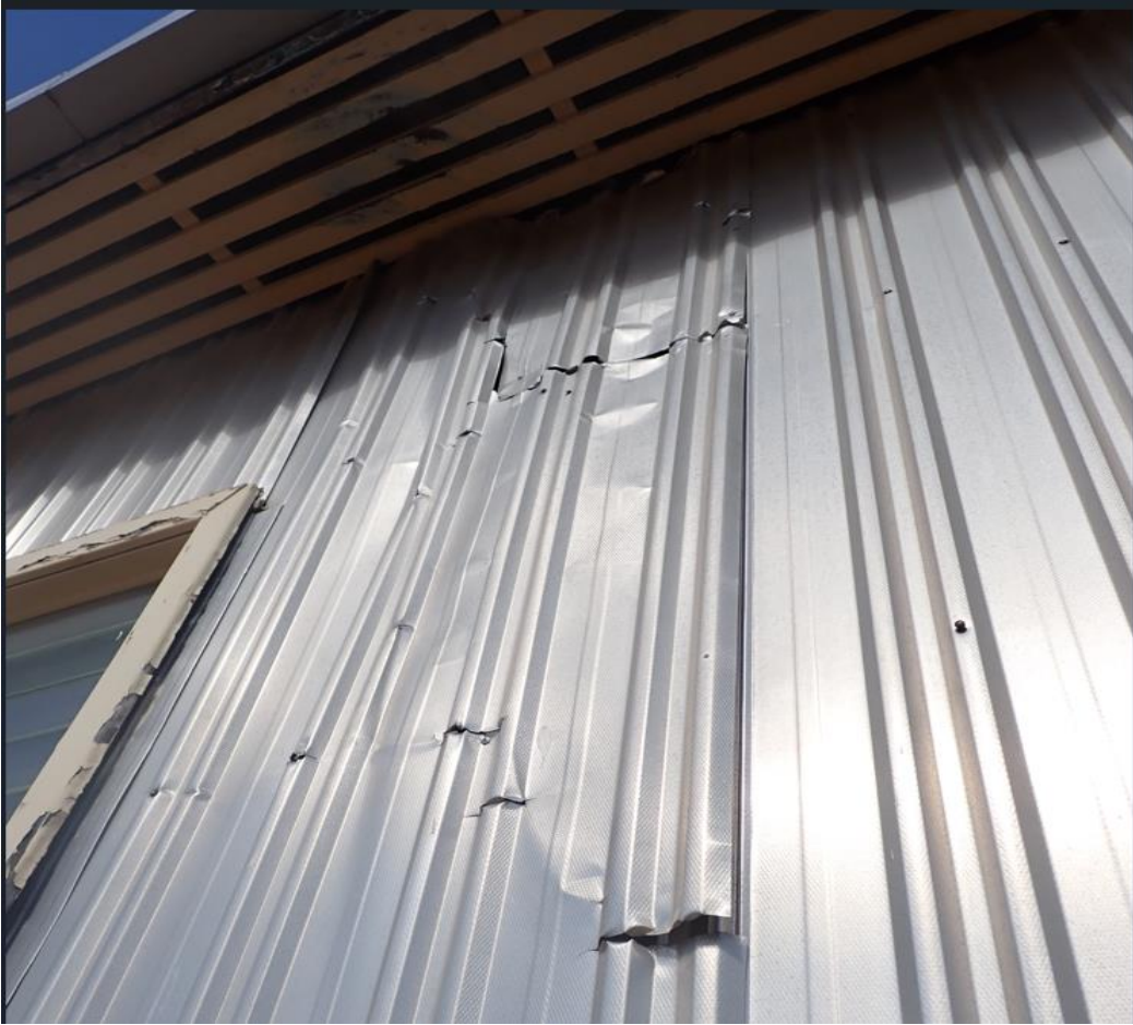
Figure 15: Damaged wall sheeting on the north side of the building.
