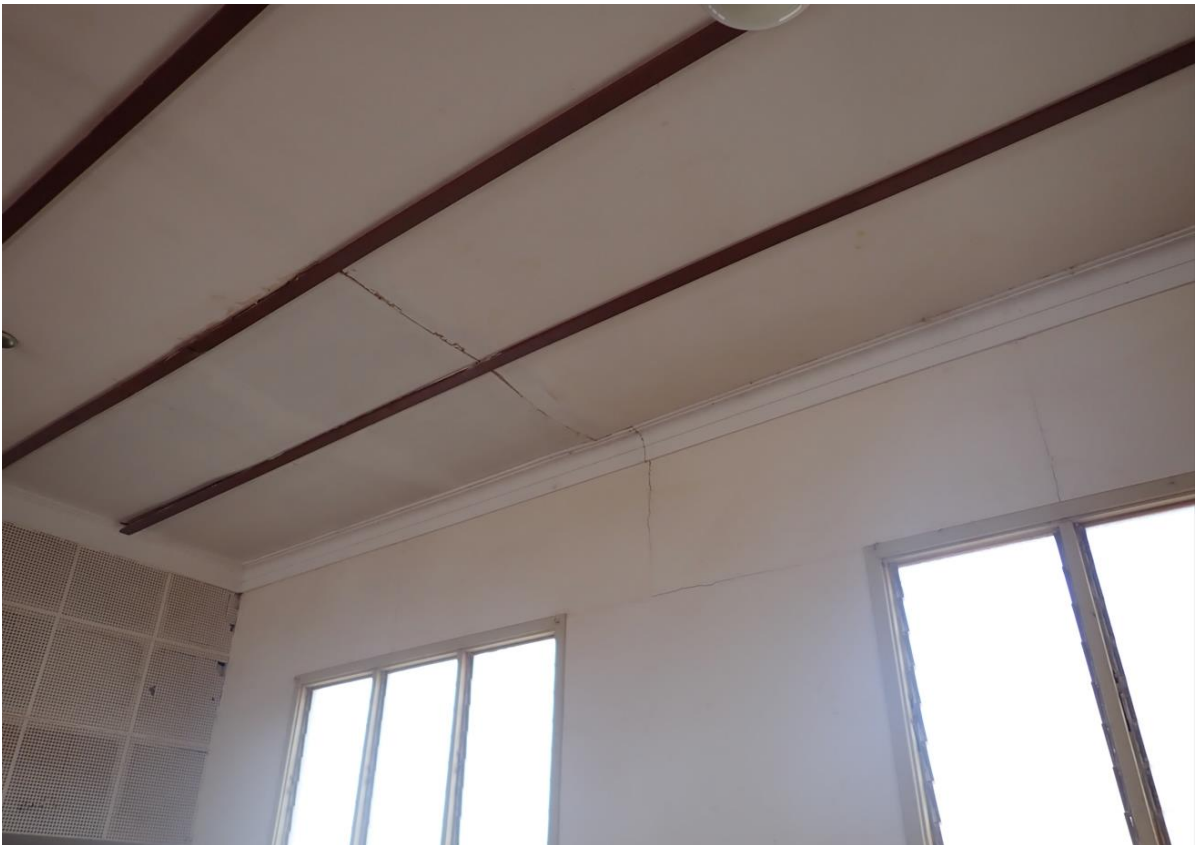
Figure 4: Wall and ceiling cracking.
