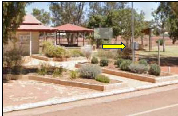
(ref: Google Maps) 3-phase power upgrade conversion to the existing switchboard located between the public toilets and verge on Fowler Street.
