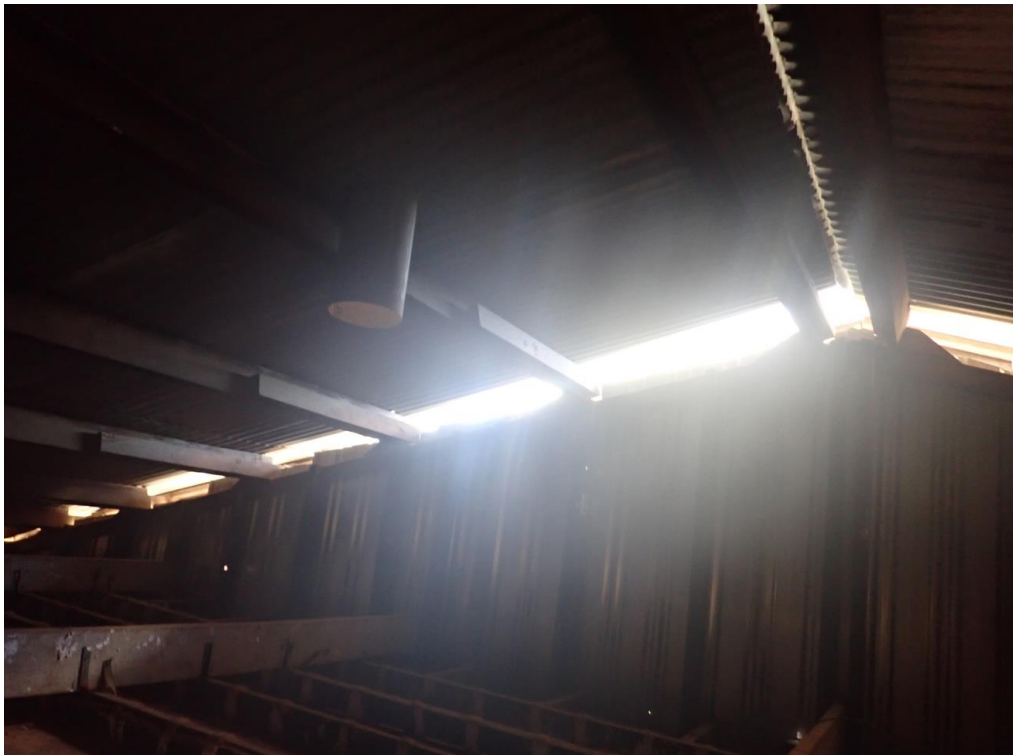
Figure 10: Roof sheeting lifting in southwest corner.
