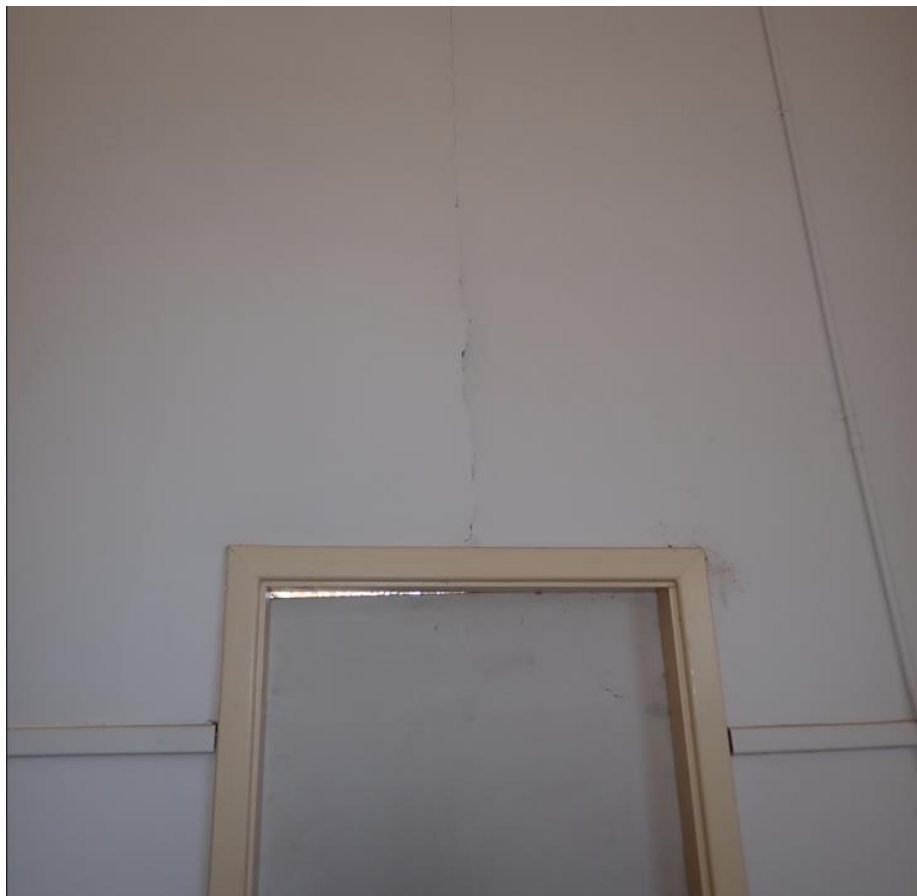
Figure 6: Wall Cracks Above Doors and Windows frame.
