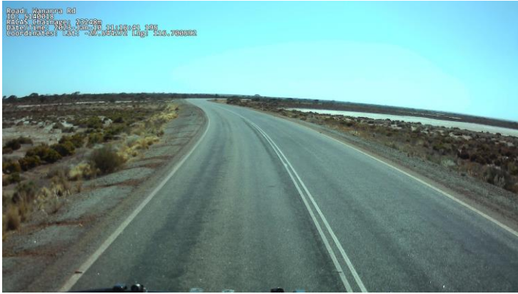
Figure 1: Wanarra Rd shoulder scour
