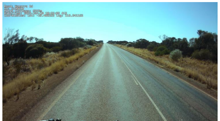
Figure 6: Wanarra Rd rutting on RHS
